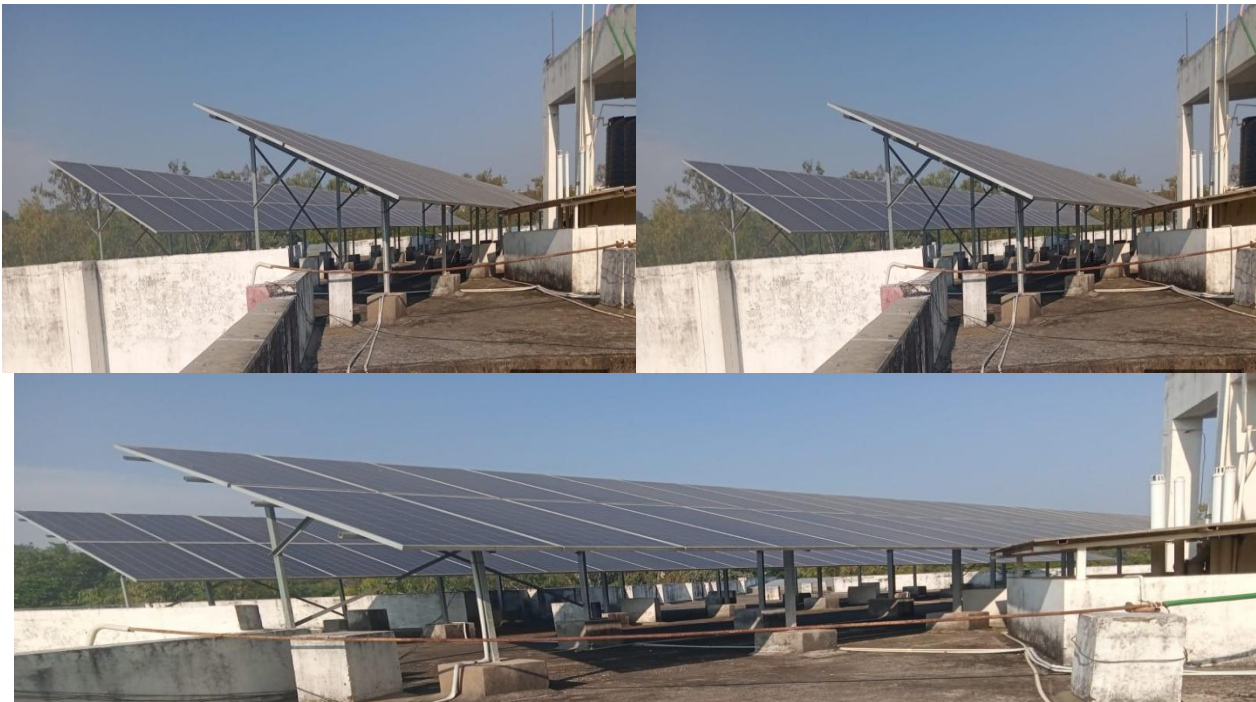
Figure 3, Solar Panel On Roof Top
